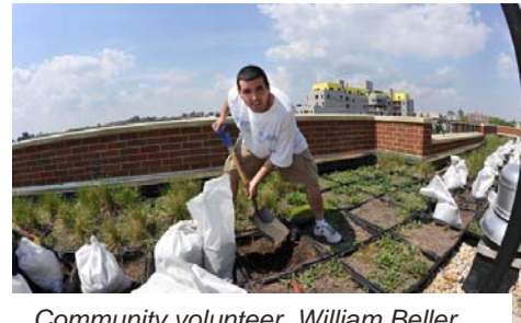
Community volunteer, William Beller, busy at work planting on Intervale Green’s roof (WHEDco)
